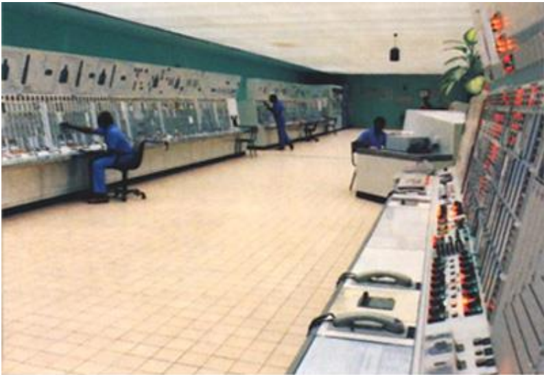
Gasco Ruwais Control room-1980s
